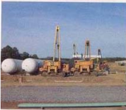
Above: Four crawlers position a 62,500-gallon propane tank on its piers at Niagara Energy’s new storage facility.
