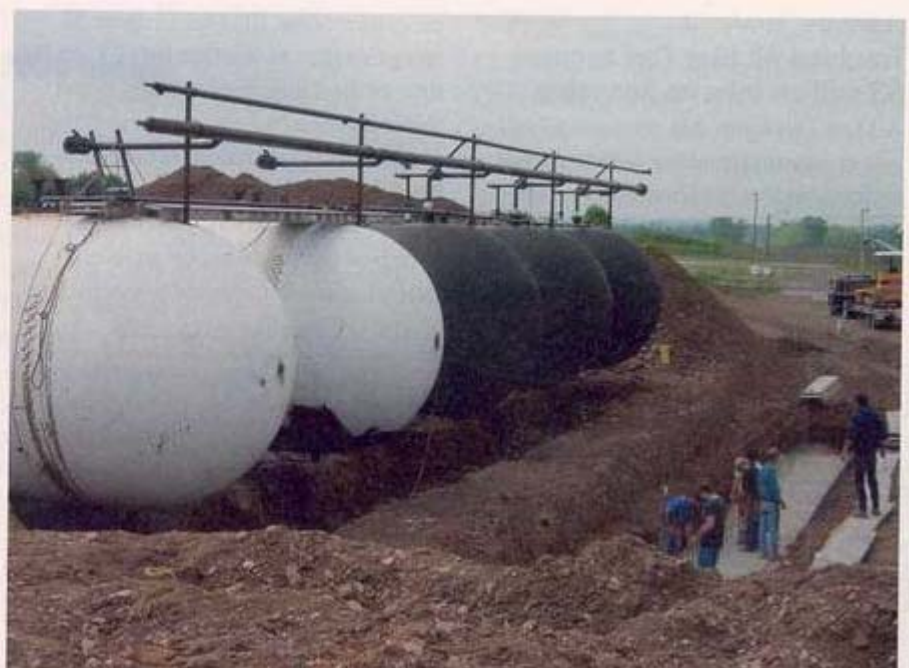
Right: All five tanks sitting in their saddles. The underground storage system will offer rail car load/unload capabilities, two transport stations and two bobtail load racks.
